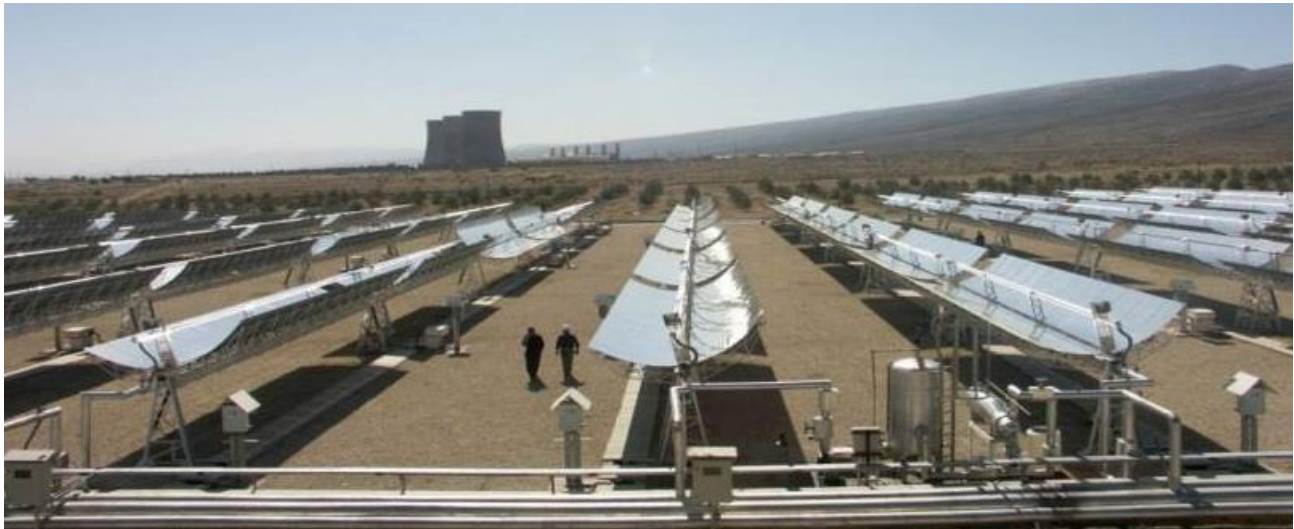
Parabolic trough collector
